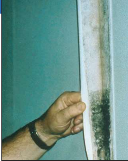
Mold growing on the back side of wallpaper.
